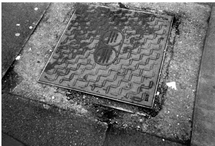
Looks like too much sand in the cement mix to me... A small hole making big trouble. Photo by Sippy Azizollah
