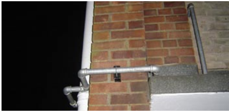
The new gas pipes attached to homes in Park Farm Close. Photo by Melanie Bruck
