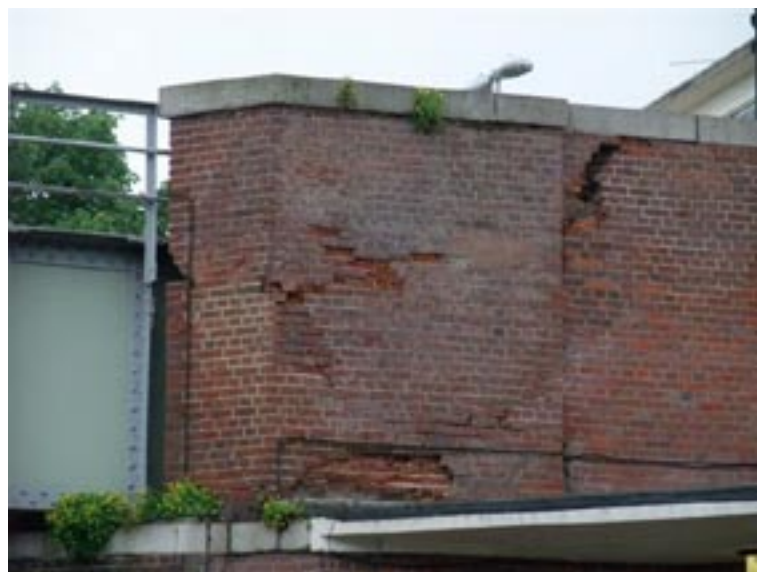
Alarming Crack Photograph by John Dearing
