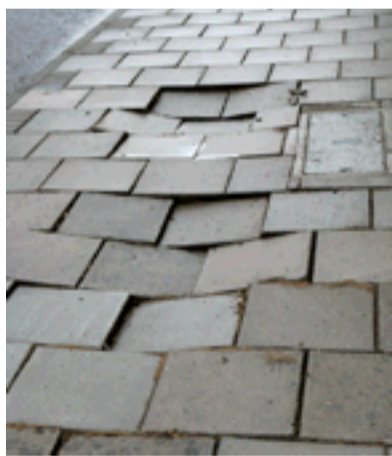
Sinking feeling: the hole in the pavement outside Whittington Court has reappeared. Photo by Neville Robinson.
