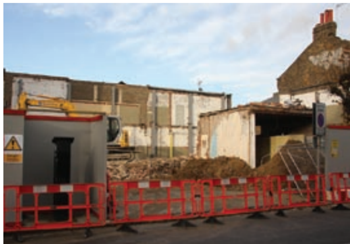
The demolition crews move into Lincoln Parade. Photo Martin Addison. Write to us at THE ARCHER, PO Box 3699, London N2 8JA, or email the-archer@lineone.net
