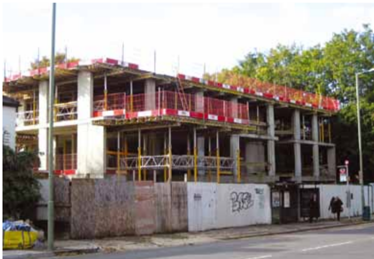
Building work has come to a halt at the site on Great North Road. Photo by Nick Young
