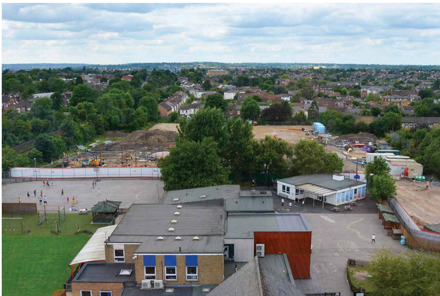
The Archer Academy building site at Stanley Field with Holy Trinity school in the foreground. Photo Mike Coles
