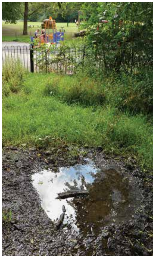
A large puddle of still water from a leak near the children's playground in Cherry Tree Wood. Photo Mike Coles
