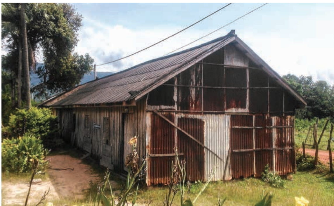
Schoolwork: The delapidated classroom in a small village near Kampot, Cambodia, that Guy's Trust hopes to renovate.
