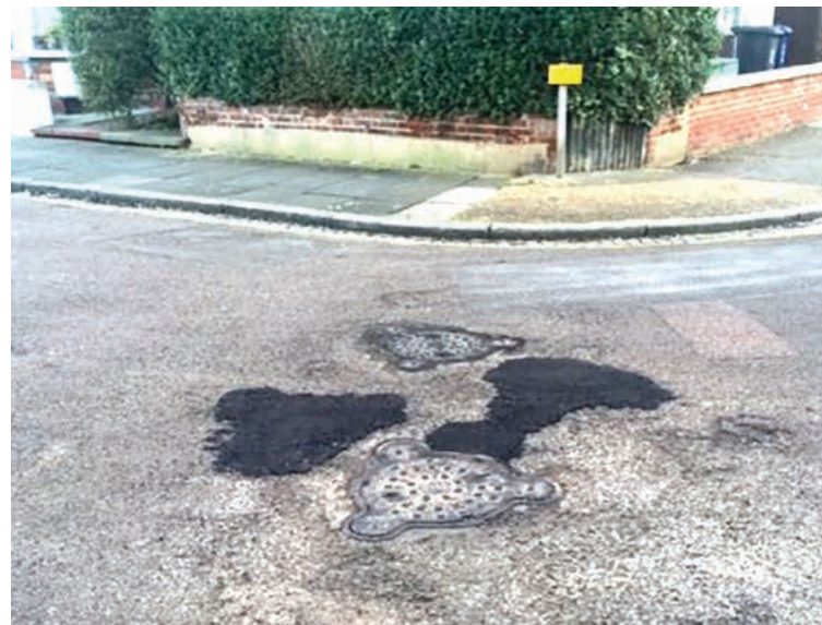
A hastily filled pothole in Beresford Road. Photo by Arjun Mittra.
