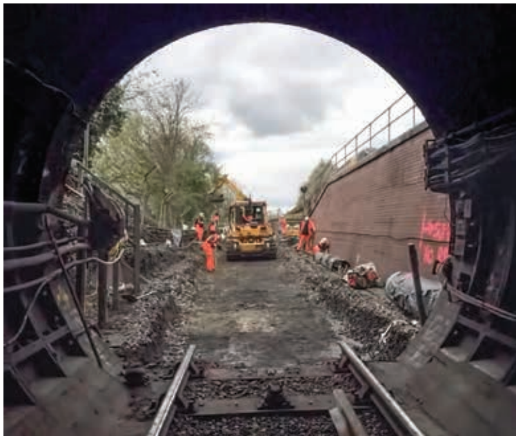
Tunnel vision: Contractors re-lay the Northern line track at East Finchley. Photo courtesy ???
