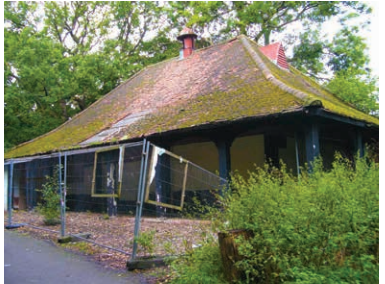
Dilapidated: The pavilion. Photo by Diana Cormack
