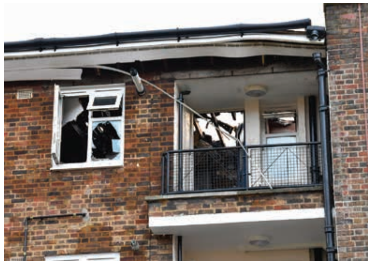
Upper floor flats completely destroyed. Photo by Mike Coles
