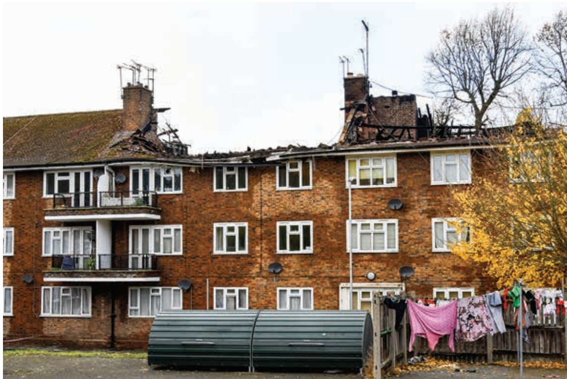
The damage to Willow House Photo Mike Coles
