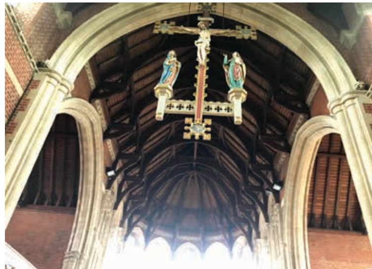
The church's hammer beam roof and exterior need repairs
