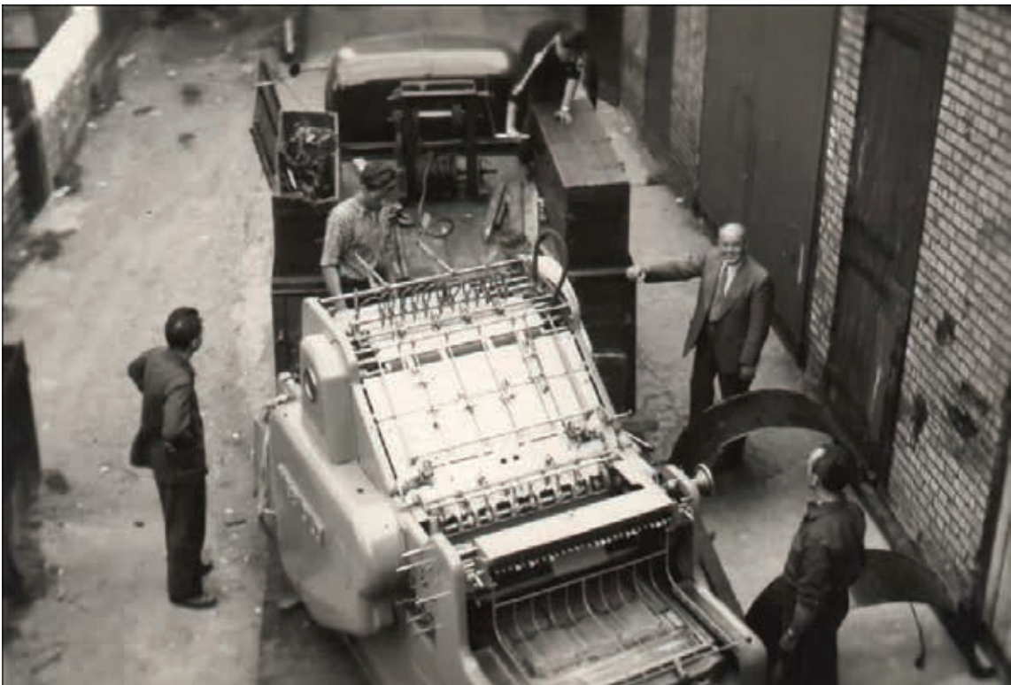
Print ready: Founder JG Bryson, centre right, watches the installation of one of the original Italian presses.
