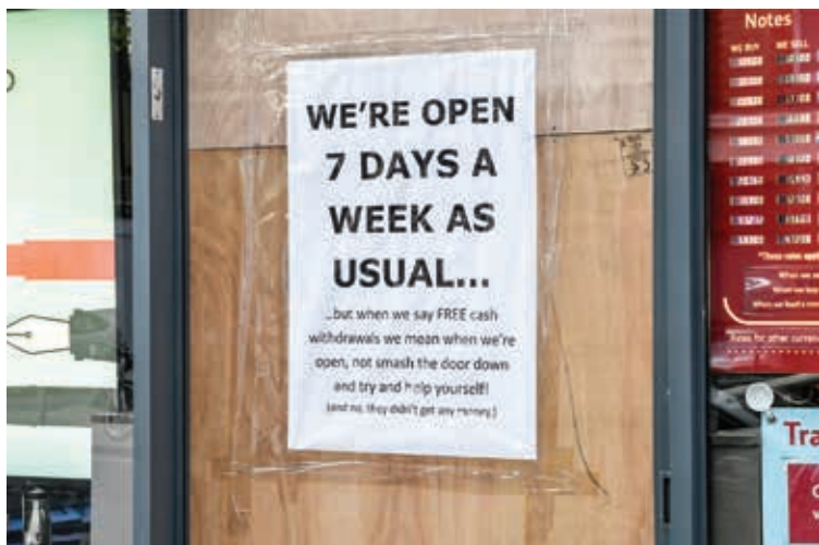
The damaged door of the Post Office. Photo Mike Coles
