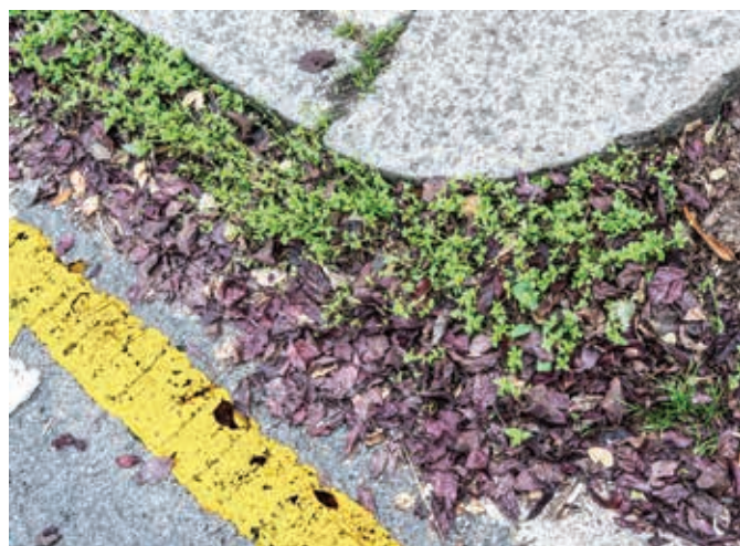
Plants growing in the uncleaned gutters Photo Mike Coles
