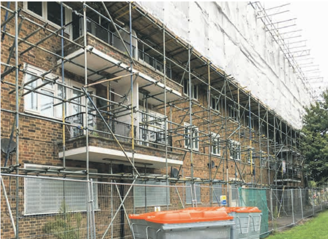
Waiting for repair: The current state of Willow House. Photo Ruth Anders
