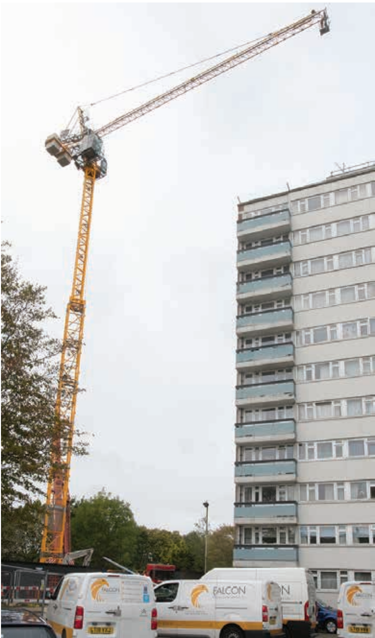
The tower crane is erected at Prospect Ring for the new block. Photo Mike Coles
