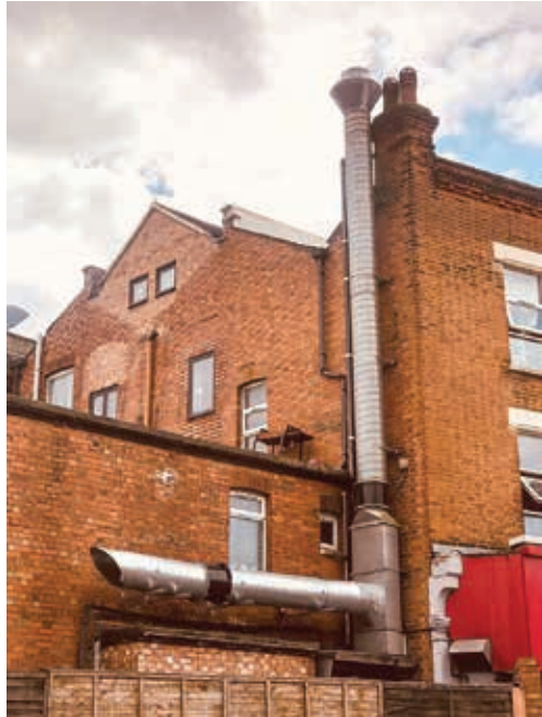
Short lived: This horizontal vent was removed from the side of the KFC restaurant in Huntingdon Road soon after being installed
