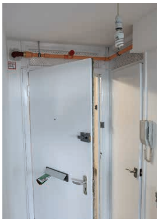
Work in progress on the new sprinkler system being installed at Prospect Ring. Photo Mike Coles
