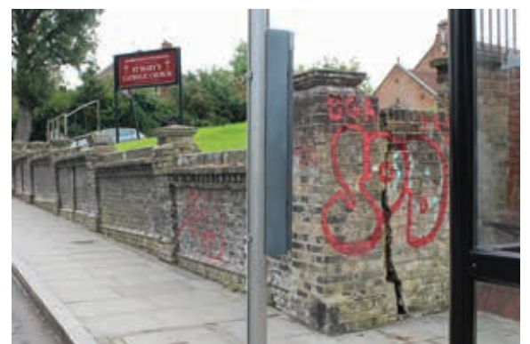
Split personality: The cracked front wall of St Mary's is in urgent need of repair.
