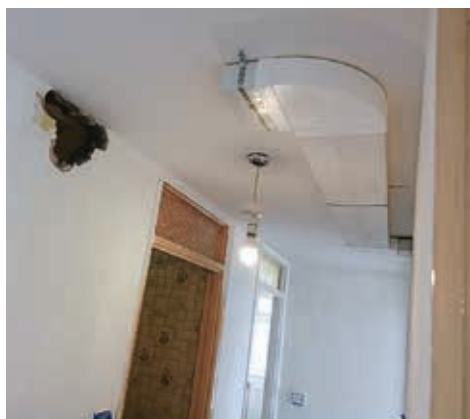
Extractor: Ceiling ducting in one Prospect Ring flat
