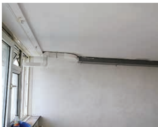
Outlet: The ducting ends at one of the flat's windows
