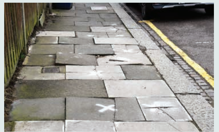
Cracked: The damaged pavement near Ann's house
