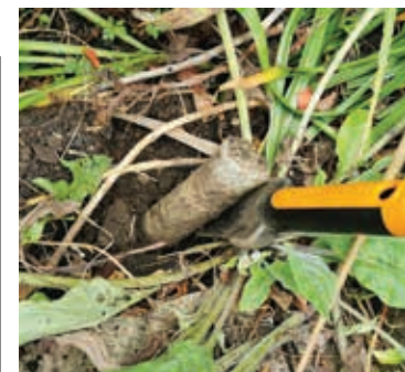
Uncovered: The cause of all the trouble
