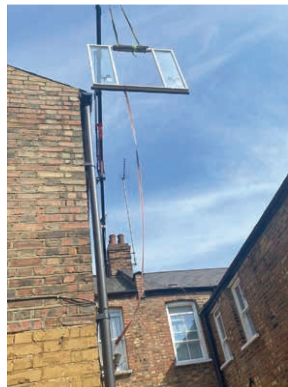
Hoisted aloft: The lorry crane lifts Fanny Petch's doors over her rooftop from the road.
