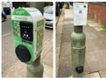
Roadside: A lamppost charging point
