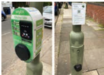
Roadside: A lamppost charging point
