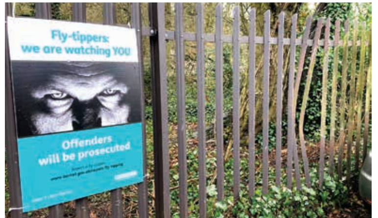
Cleared: A warning sign next to the damage to the fence where the skip used to be in Brompton Grove. Photo Mike Coles.
