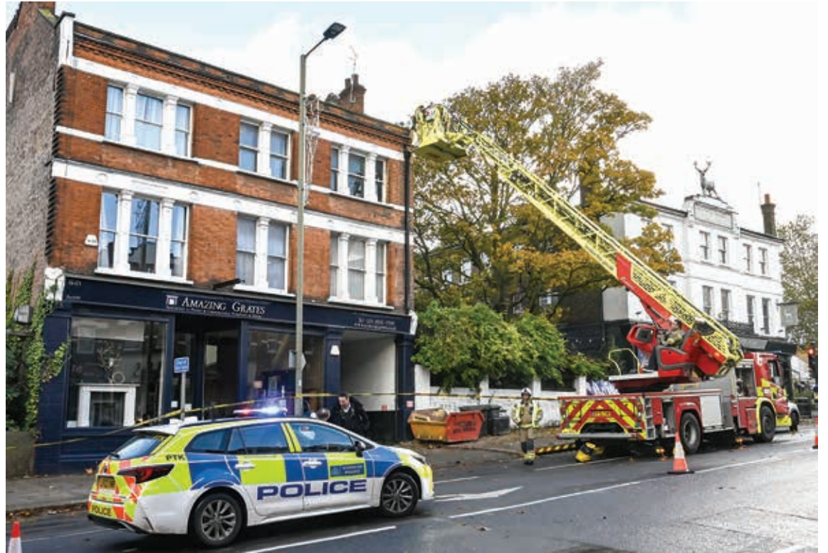
Long drop: Fire crews make safe the broken masonry and brickwork above the Amazing Grates shop. Photo Mike Coles
