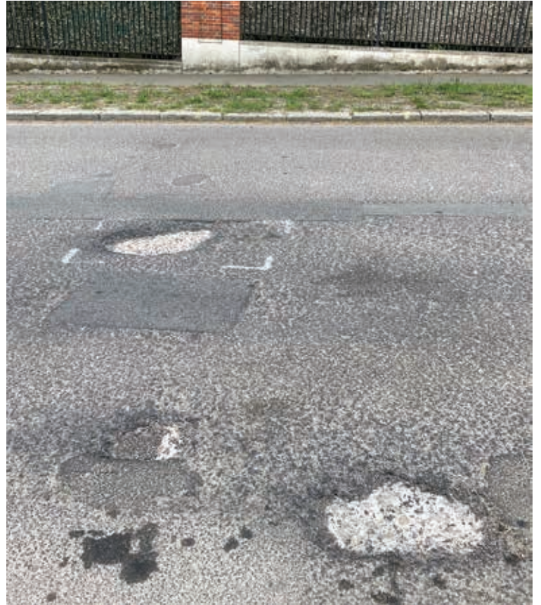
Obstacle course: The Bishops Avenue is pitted with potholes
