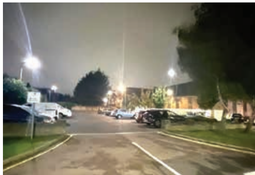
Before and after: Norfolk Close was in semi-darkness (above) until its car park lights were fixed
