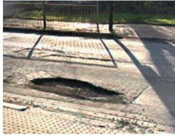
Hazard: The East End Road pothole, since filled in
