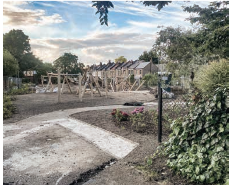
Taking shape: New equipment is being installed in Market Place Playground. Photo Samantha Haycock
