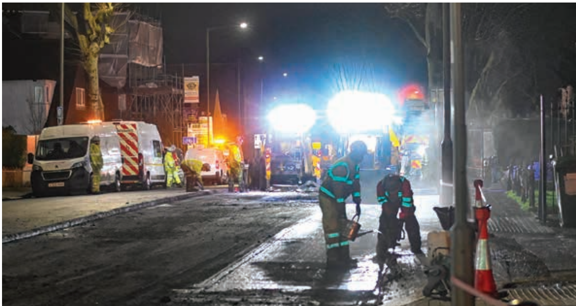
Night work: Resurfacing machinery and crews move up the High Road after evening rush hour. Photo Mike Coles
