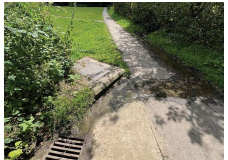
Running water: The leak across the path. Photo Mike Coles
