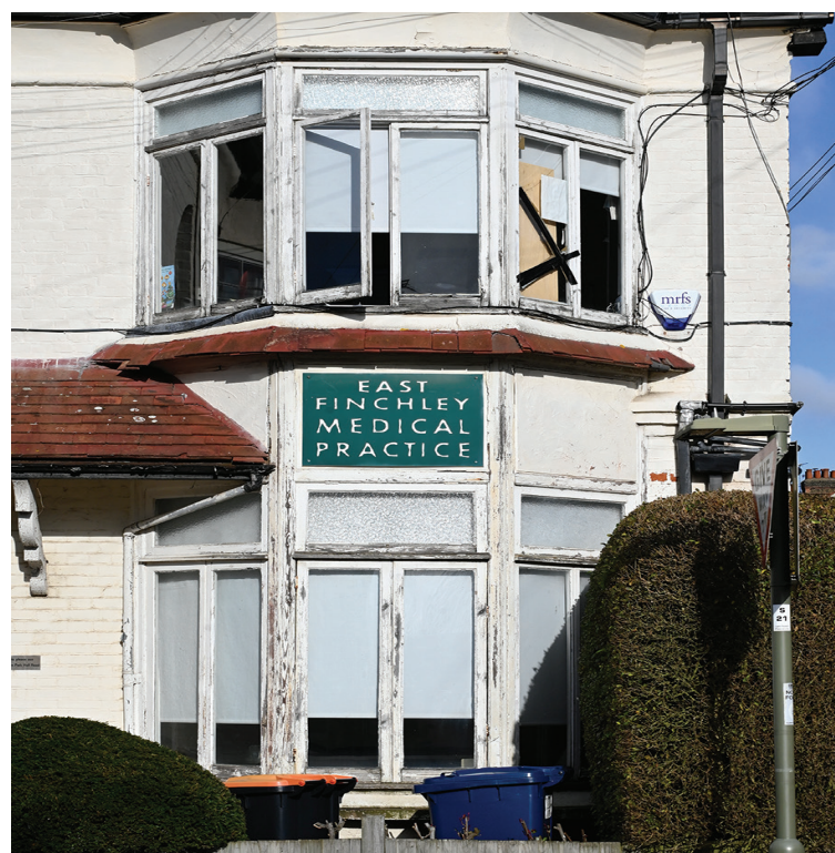
Needs attention: Peeling paint and a broken window mark the external appearance of the East Finchley Medical Practice. Photo Mike Coles
