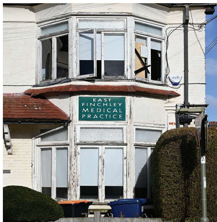
Needs attention: Peeling paint and a broken window mark the external appearance of the East Finchley Medical Practice. Photo Mike Coles
